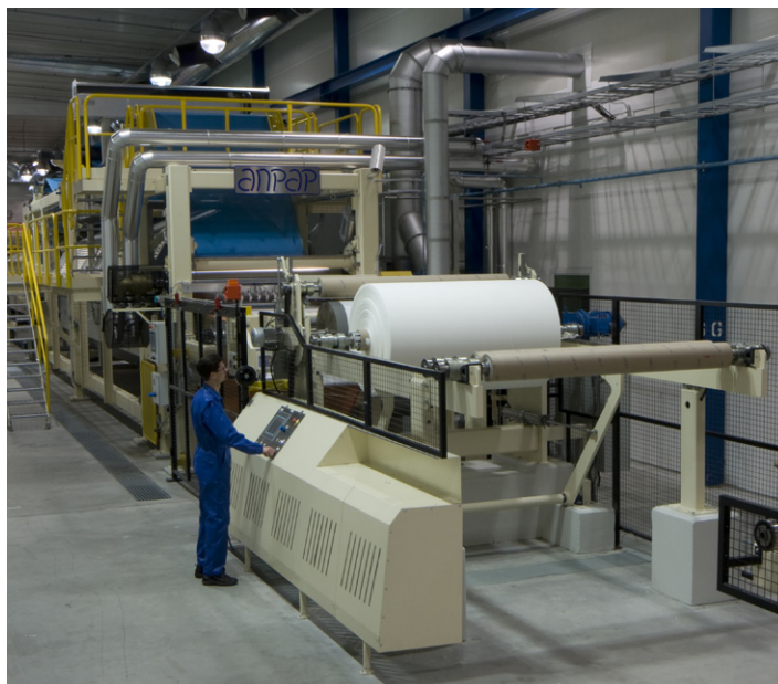
A leading airlaid technology company, Anpap, has delivered a complete airlaid production line to Lacell Oy's new nonwovens plant in Iitti, Finland.
